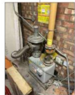
GAS METERS & ISOLATION POINT.
