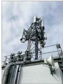
TELECOMS ARE ROOF MOUNTED ON PLANT ROOM.
