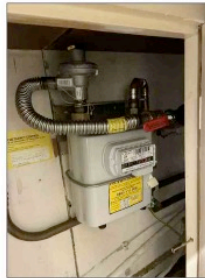
GAS METERS & ISOLATION POINT.
