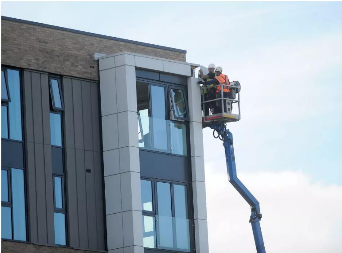
📸 Cladding is removed from a tower block in Wythenshawe (Image: Manchester Evening News)
